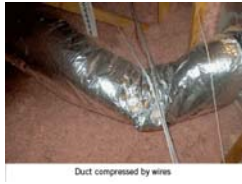
Duct compressed by wires
