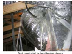
Duct constricted by bend leaving plenum
