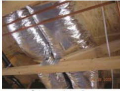
Ducts compressed into small space
