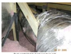
Duct constricted by bend over truss web.
