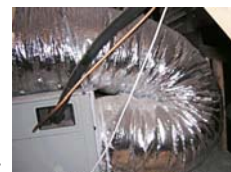
Radius of bend less than duct diameter
