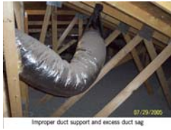
Improper duct support and excess duct sag
