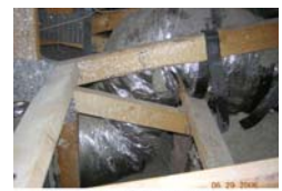
Duct constricted by two bends leaving plenum
