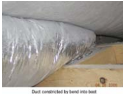
Duct constricted by bend into boot
