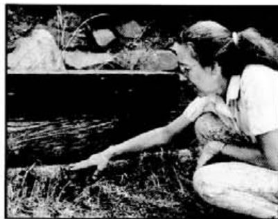
The author is shown with a Camponotus modoc infestation in railroad ties. Notice the debris between the ties.
