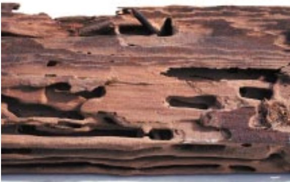
Fig. 6. Carpenter ant galleries (note sawdust fragments in lower right quadrant).
