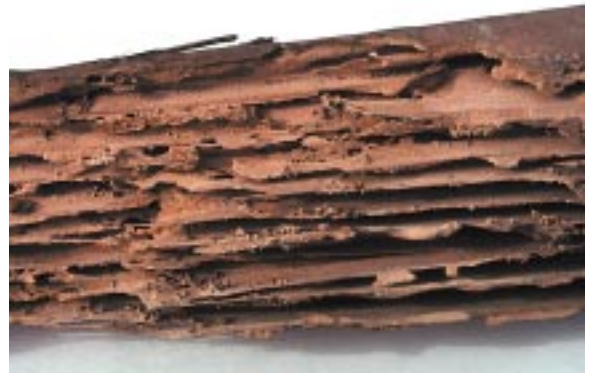
Fig. 2a. Damage and fecal pellets of dampwood termites.
