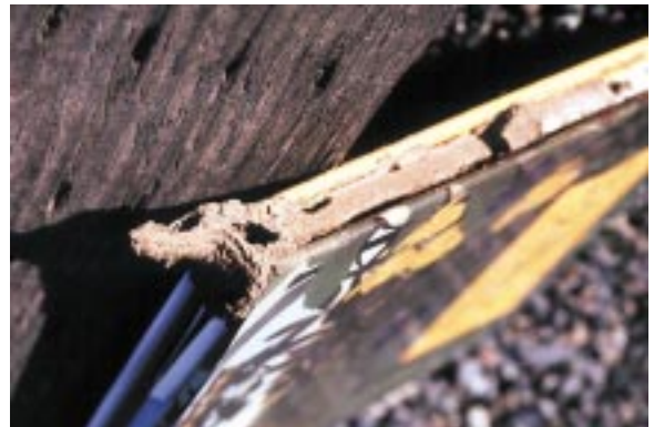
7c. Subterranean termite mud tubes.
