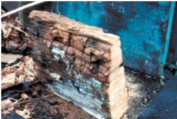
Fig. 1. Wood decay fungi in a support beam damaged by rain leakage.
