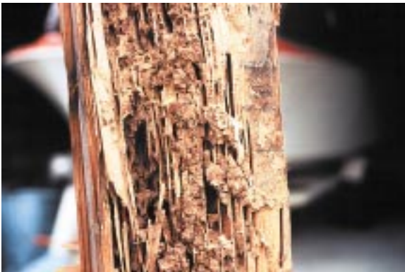
Fig. 7b. Subterranean termite damage.
