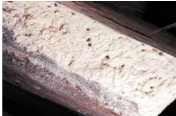
Fig. 4d. Lyctid beetle damage.
